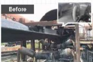
Forcibly pressing the floating belt with the wheels caused damage and mistracking of the belt.
